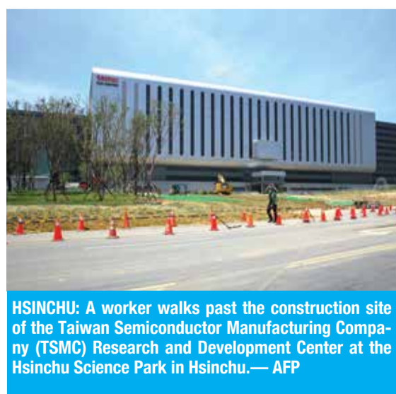
HSINCHU: A worker walks past the construction site of the Taiwan Semiconductor Manufacturing Company (TSMC) Research and Development Center at the Hsinchu Science Park in Hsinchu. - AFP
